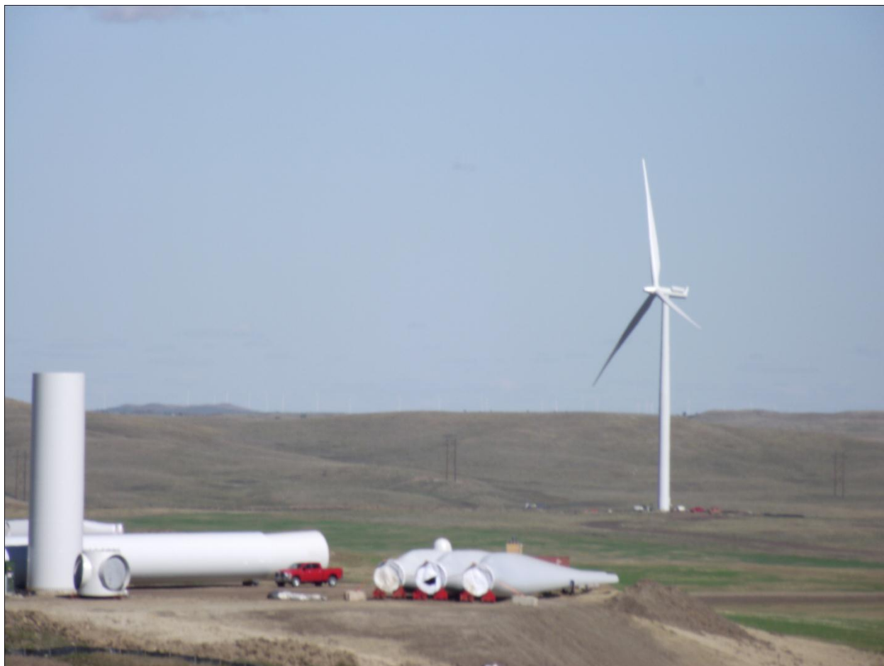
One of Minnesota Power's wind generators on the Bison Wind Farm
