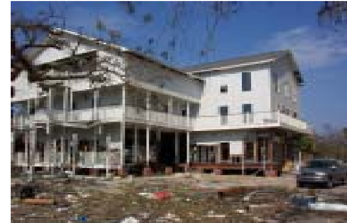
W. G. Yates and Sons Construction Company's Main office in Biloxi, Mississippi after Hurricane Katrina hit. The entire first floor was completely destroyed. Regardless, they were among the first business in the area to reopen.
